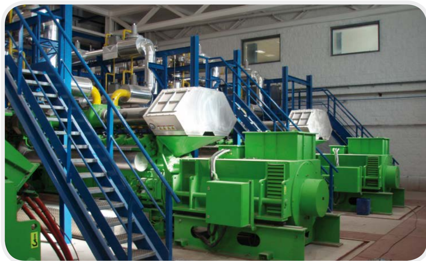
6 MWe synthesis gas engine generator room
