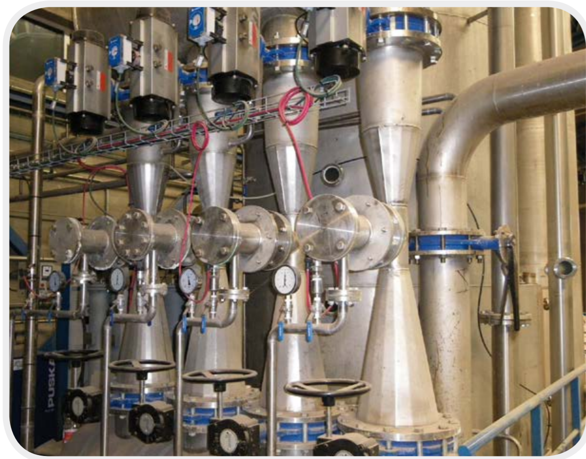
Syngas cleaning system
