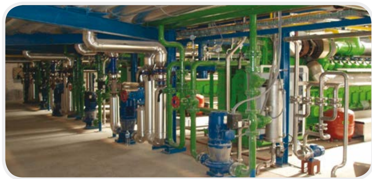
Heat recovery units for the production of hot water
